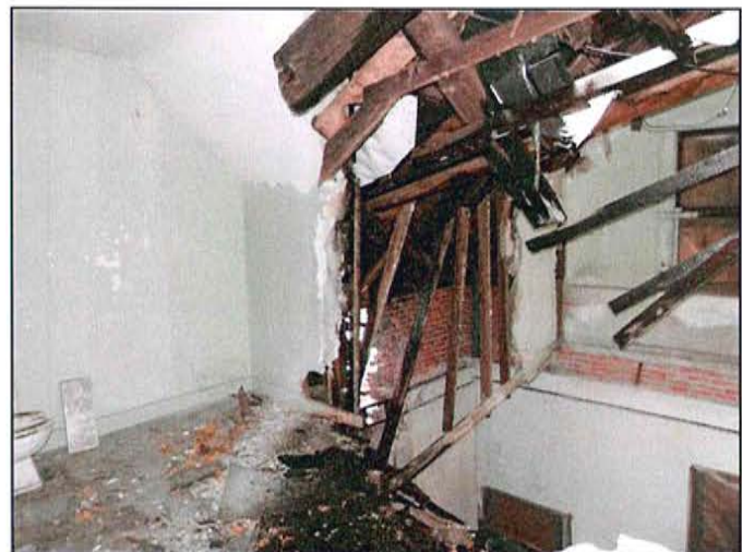
PHOTO 22: 3 rd Floor, collapsed stairs, northwest
