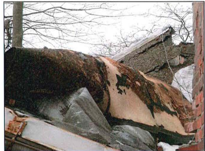
PHOTO 58: Roofing on collapsed carport
