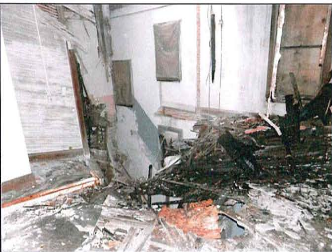
PHOTO 23: 2 nd Floor, collapsed stairs, northwest
