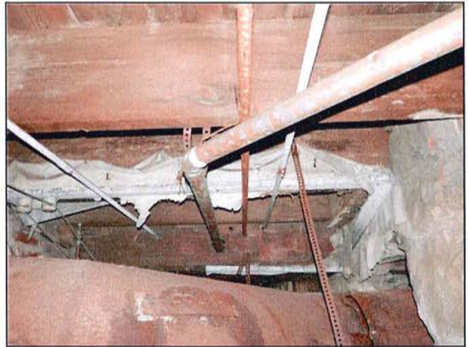
PHOTO 38: Residual insulating paper in basement hall
