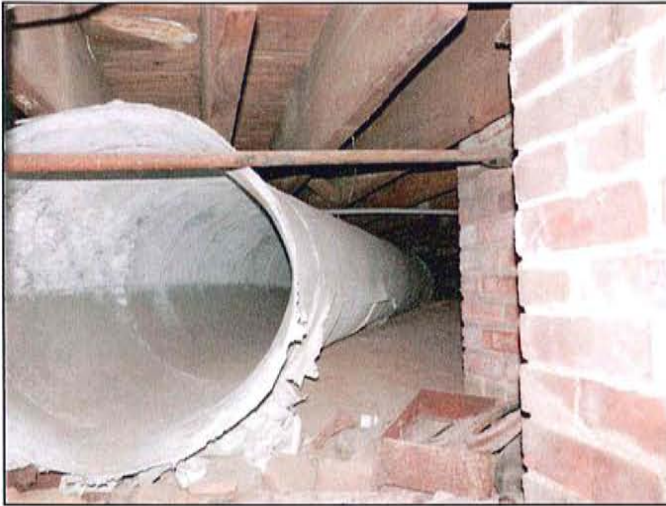
PHOTO 37: Insulating wrap on 24" basement duct
