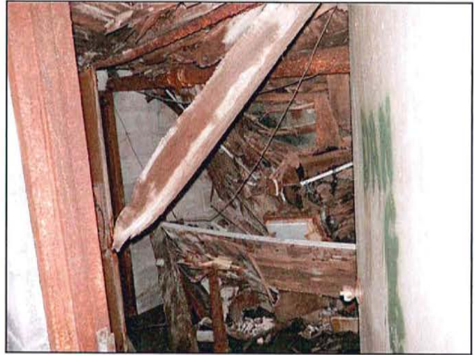
PHOTO 32: Collapsed basement room, northeast
