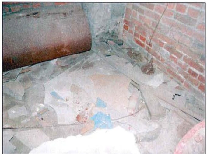
PHOTO 36: Transite debris in basement crawl space
