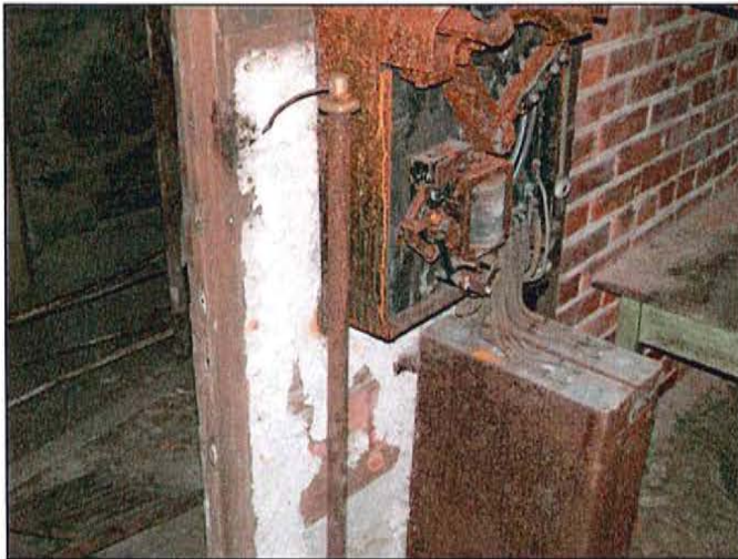
PHOTO 39: Electrical equipment insulating board
