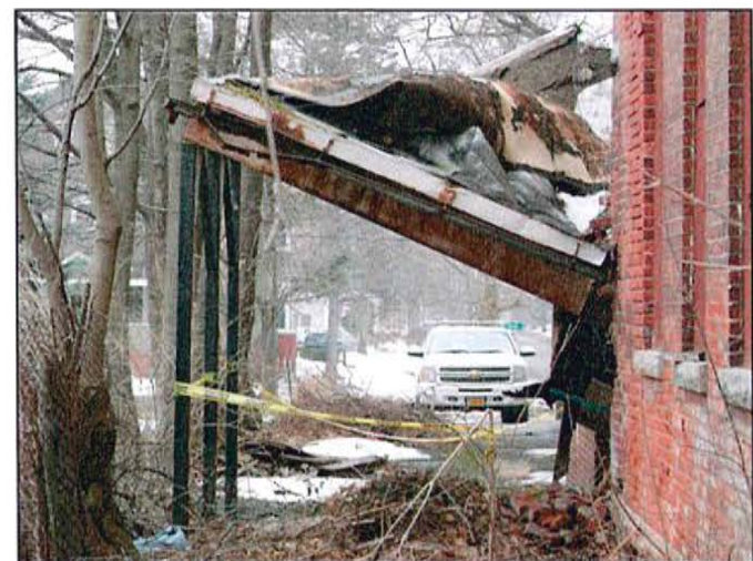
PHOTO 6: Collapsed carport at south entrance
