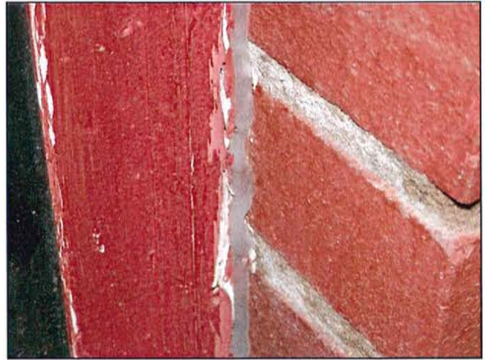
PHOTO 56: Exterior brick caulking type 2
