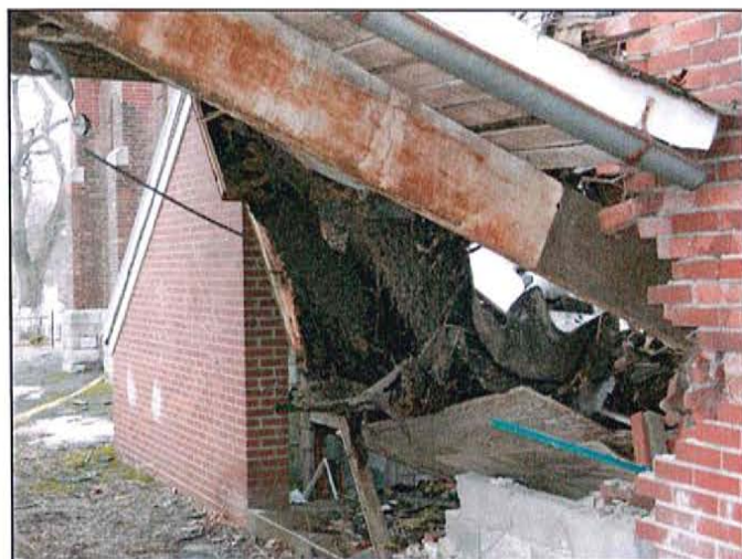
PHOTO 5: Collapsed roofing at south entrance
